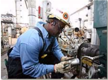
Bobby Manning, who works in the coker unit at the Pascagoula Refinery, uses a handheld computer to monitor temperatures, pressures and vibrations. Chevron introduced this device in 2004 to improve reliability.
